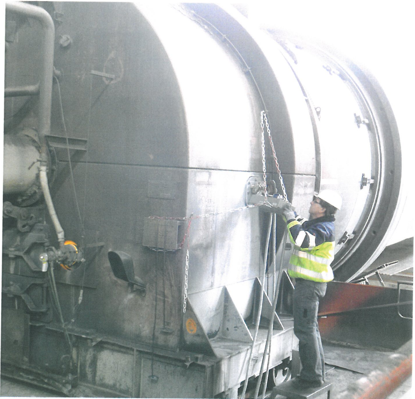
Pic. 9: Thermal imaging camera - mounted on the side of the kiln hood
